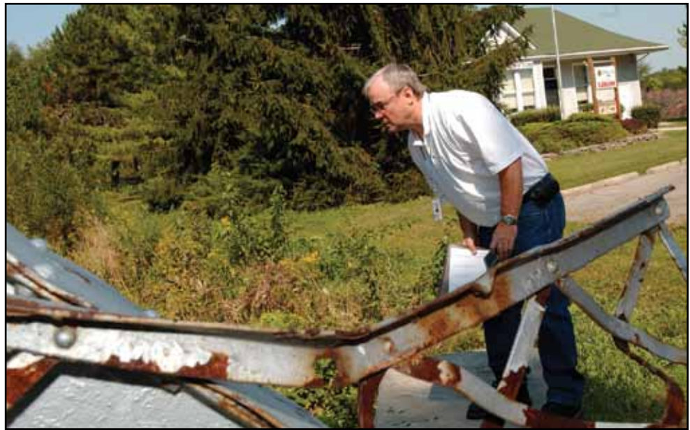
Paul Ogiba, a FEMA representative, examines damage to a bridge after flash floods swept through. FEMA conducts Preliminary Damage Assessments (PDA) to communities affected by disasters. John Ficara/FEMA
