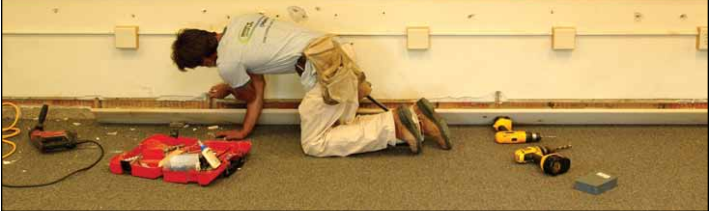
A carpenter makes repairs on a classroom that was flooded at Central Middle School in downtown Findlay. FEMA programs provide money to help repair public buildings that have been damaged. John Ficara/FEMA
