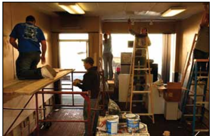
Students from the University of Findlay help to repair “Java Station,” a local coffee house that was damaged by flooding in downtown Findlay. John Ficara/FEMA
